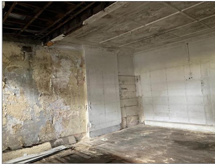
Figure 22: Looking towards the remnant chimneypiece on the west end of the shop. Note the cracked and peeling plasterwork to the walls and the missing ceiling to the front.
