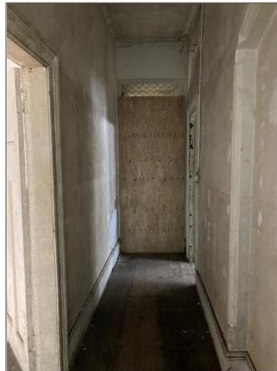
Figure 26: Hallway, looking towards a blocked entry.
