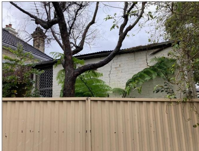
Figure 17: The eastern elevation of the rear wing as it extends from the principal building.
