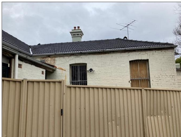
Figure 15: Eastern elevation of the principal building showing non-original concrete tiles.
