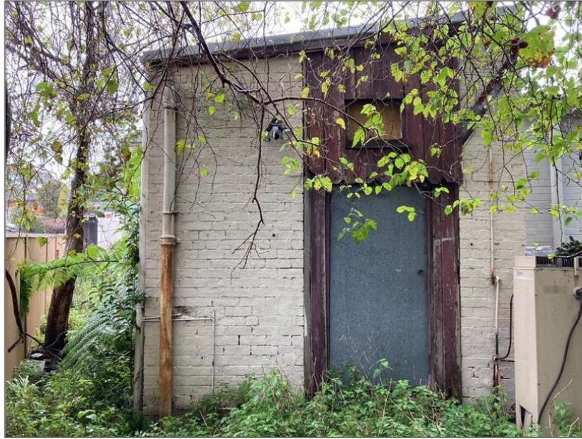
Figure 18: The rear elevation of the rear wing, showing a later metal door.
