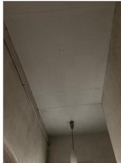
Figure 27: Hallway ceiling, showing non-original plasterboard.
