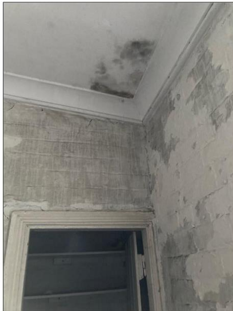
Figure 33: Close-up view of the kitchen ceiling showing mould damage.
