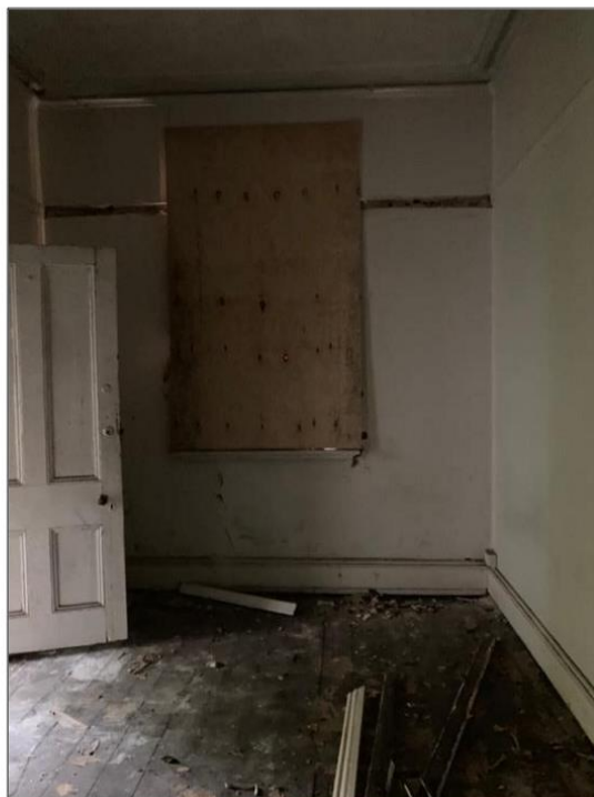
Figure 30: Living room, looking towards a blocked window opening.
