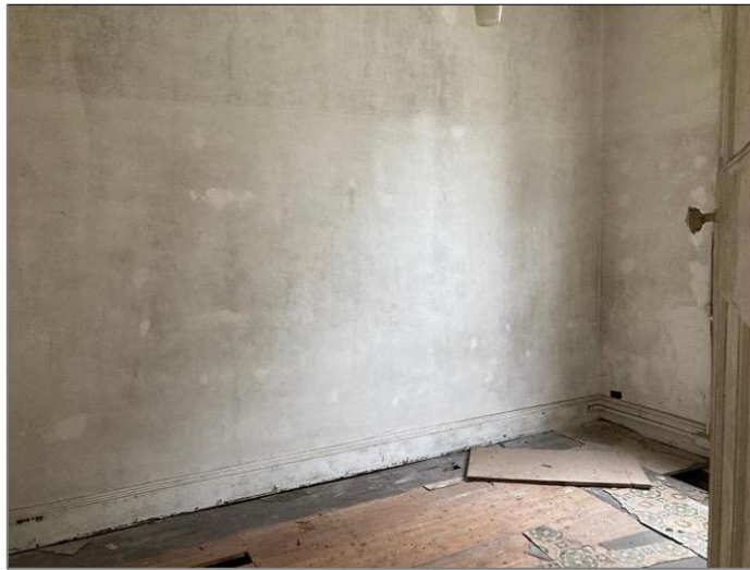
Figure 29: The bedroom showing a timber floor, with sections missing.
