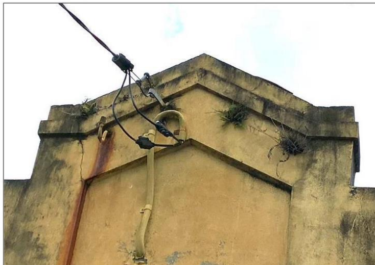
Figure 11: Close-up of the parapet showing cracks and vegetation.
