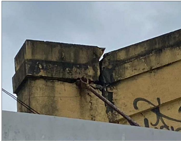
Figure 12: The fractured parapet wall on the eastern elevation.
