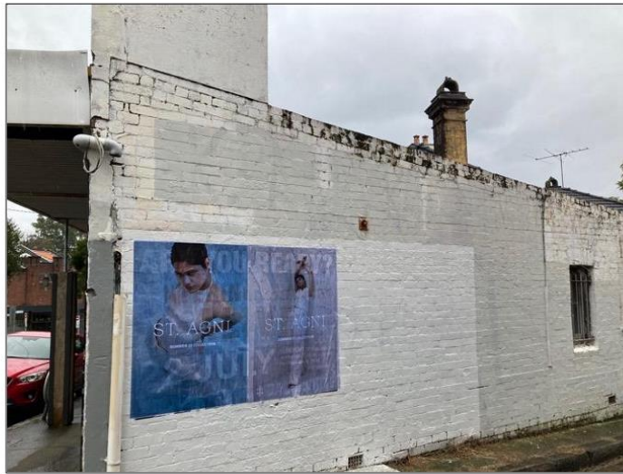
Figure 14: End of the parapet wall as viewed from Jubilee Lane. Note the cracked brickwork.
