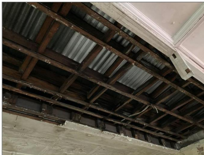
Figure 23: Close-up view of a section of missing ceiling.
