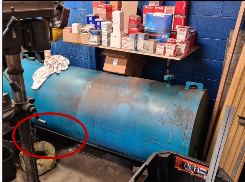
PHOTOGRAPH 4: AST WITH STAINING
