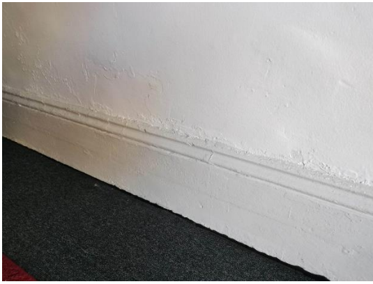
Figure 4-15: Skirting and damp damage to plaster on ground floor of 77 Crown Street. Source: Curio 2023
