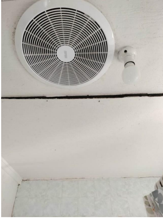
Figure 4-33: Damaged ceiling in bathroom of 75 Crown Street. Source: Curio 2023
