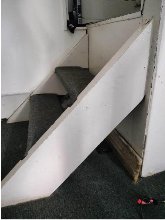
Figure 4-37: Added flight to bottom of stairwell. This area is damp to the touch with visible mould. Source: Curio 2023
