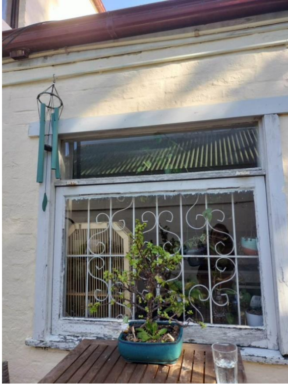
Figure 4-41: Back window of annex. Source: Curio 2023
