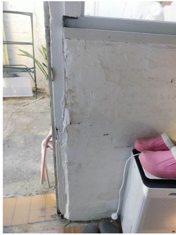
Figure 4-40: Rear door of annex with access into rear yard. Bricks are cracked and inconsistent. Source: Curio 2023
