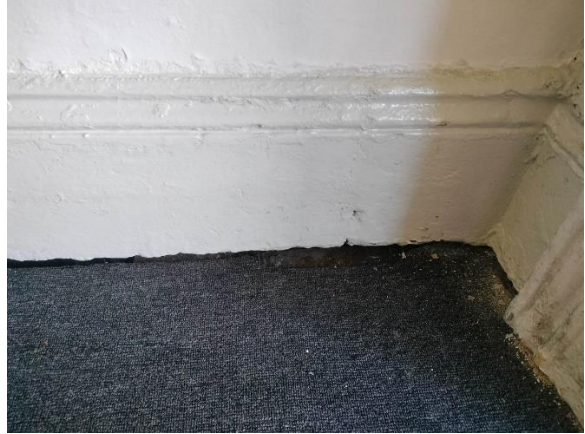
Figure 4-34: Damp damage and wet carpet near front door of 75 Crown Street. Source: Curio 2023
