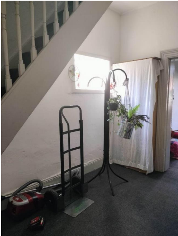
Figure 4-35: Backroom and stairwell within 75 Crown Street. Carpet in this room was damp and musty. Source: Curio 2023
