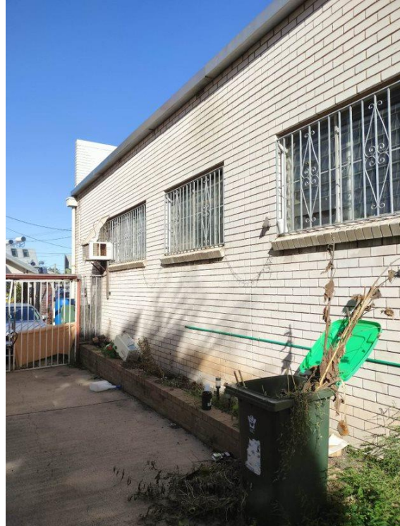
Figure 4-44: Northern wall of warehouse taken from yard of terrace, facing southeast. Source: Curio 2023
