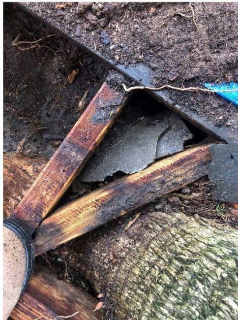
Plate 6: Image showing the asbestos found. P. Vezgoff.
