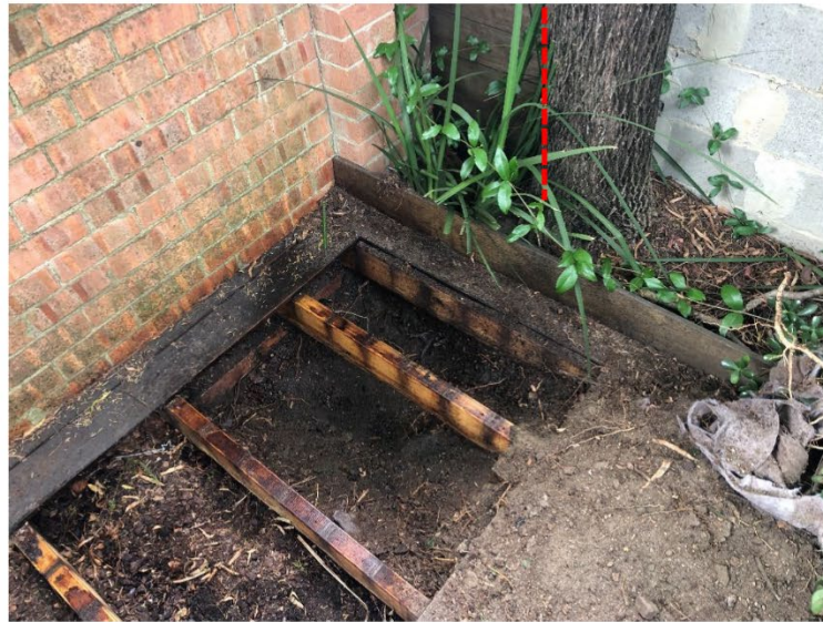
Plate 9: Excavations near Tree 2 revealed no roots however pending the survey this tree may require removal. The possible boundary is located by the red line based on the existing join in the fence. P. Vezgoff.
