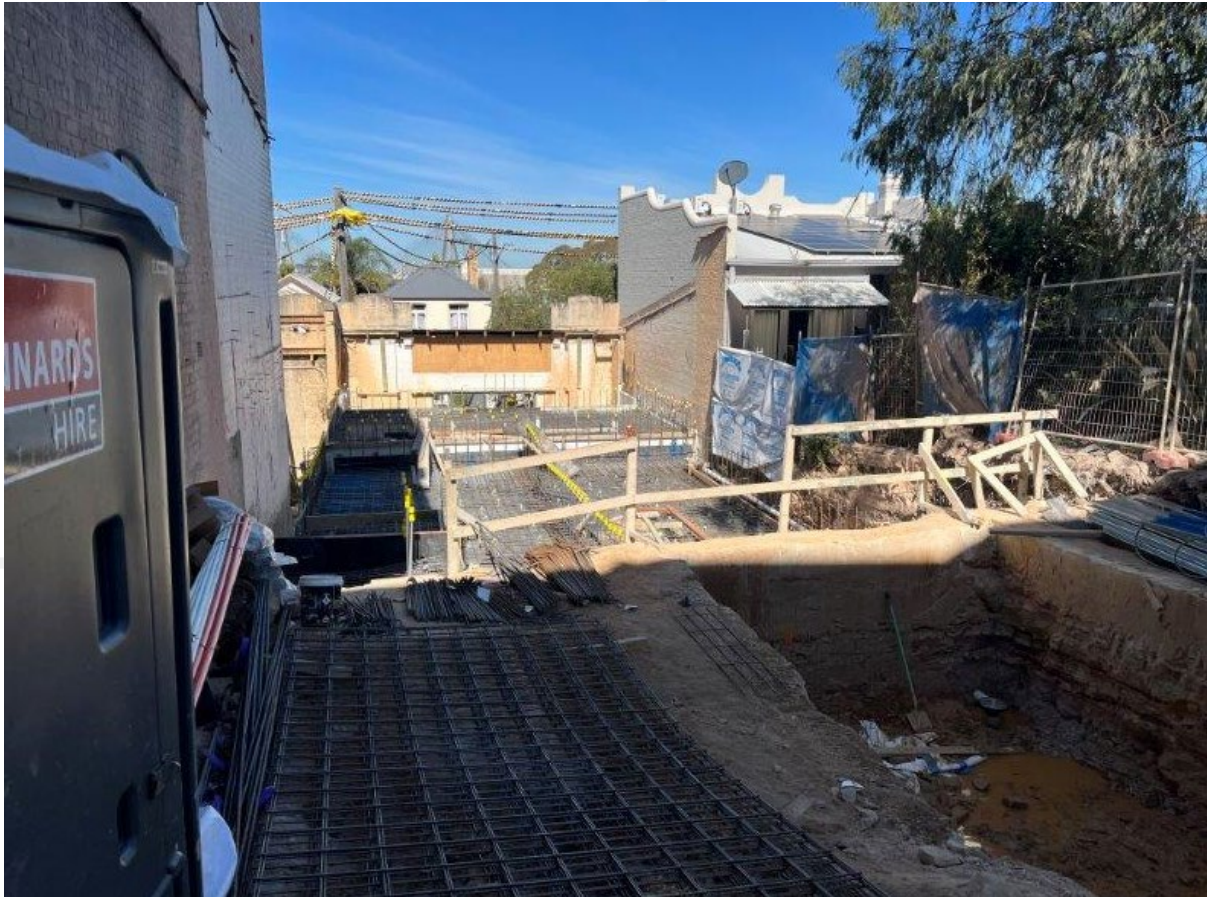
Image 1: showing removal of original roof, columns and rear wall behind the retained Beattie Street façade in the background, removal of original slab and new lowered basement level centrally located within the site and new pit for car stacker in the foreground adjacent to Little Llewellyn Street.
