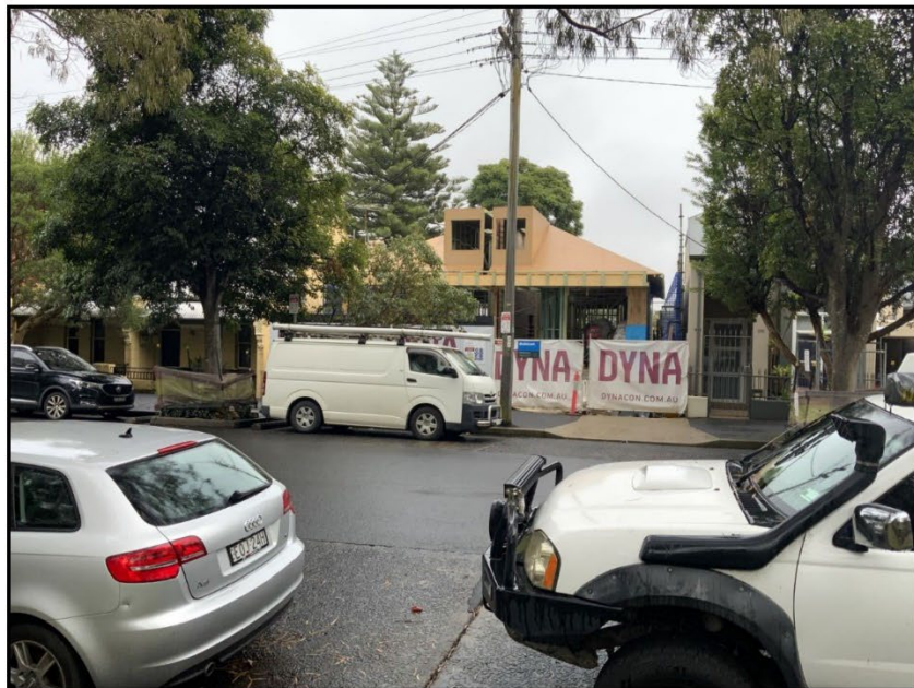
Figure 3: Subject site as viewed from Norton Street during construction, noting the casual observer is unable to discern whether the property consists of strata attached dual occupancies or torrens title semi-detached dwellings
