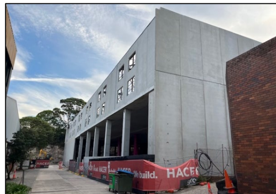
Figure 4: Photo of rear(east) of building under construction (as viewed from rear private lane)
