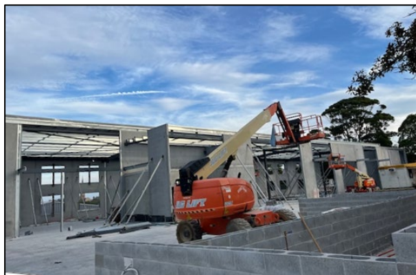
Figure 3: Photo of building under construction (as viewed from north on Catherine Street)
