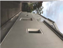
new roof gutter to be connected to existing downpipe to front of house
