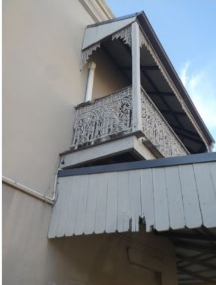
Vertical timber spandrels to veranda and awning with minor rot
