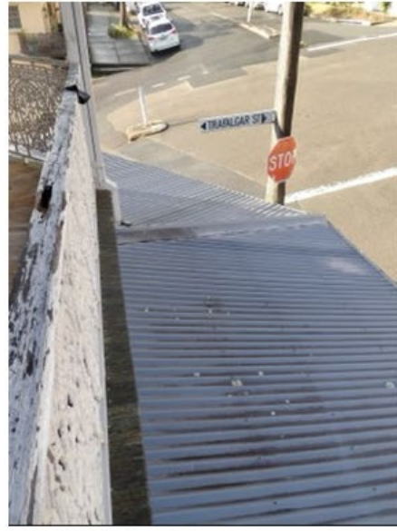
Weathered handrail, roof of awning, south side of building
