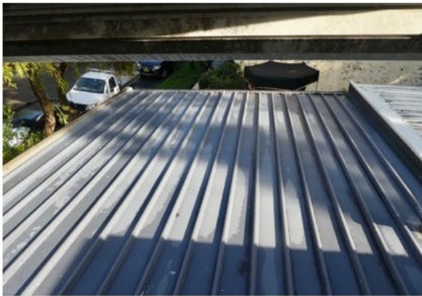
Roof of the kitchen/ family room, from the rear first floor bed room
