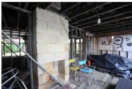
Figure 31 – Looking north-east through the cottage. There is evidence that the stone fireplace was originally plastered with timber mantles.
