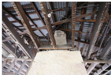
Figure 32 – Remains of chimney breast (the chimney has been demolished above the roof line).
