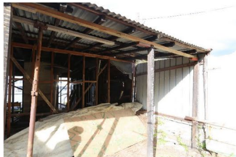
Figure 26 – View of rear skillion roof extension to the northern portion of the cottage.
