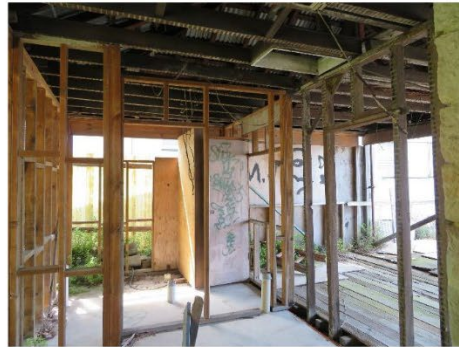
Figure 28 – Looking west through cottage, with new concrete floor slab a timber studs.
