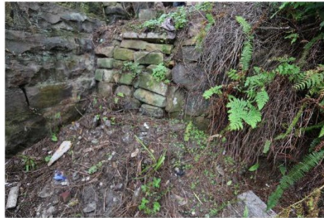
Figure 40 – Stone retaining wall on the western boundary of the site. It is assumed that a stair may have been previously located here.
