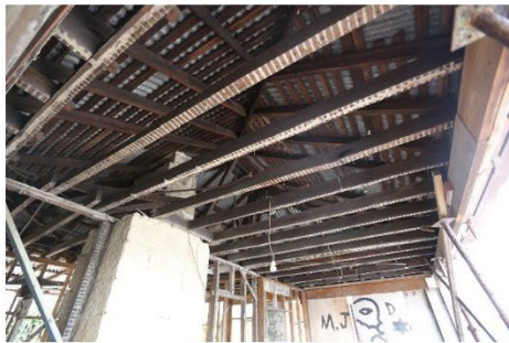
Figure 35 – Exposed roof beam and rafters, with earlier corrugated iron sheeting. Some of the roof beams appear to be hand hewn.
