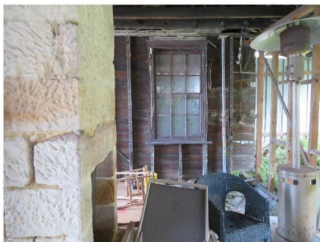
Figure 29 – Looking west across the cottage. This is the only remaining original joinery. One piece of the architrave remains along the top of the window although in poor condition.
