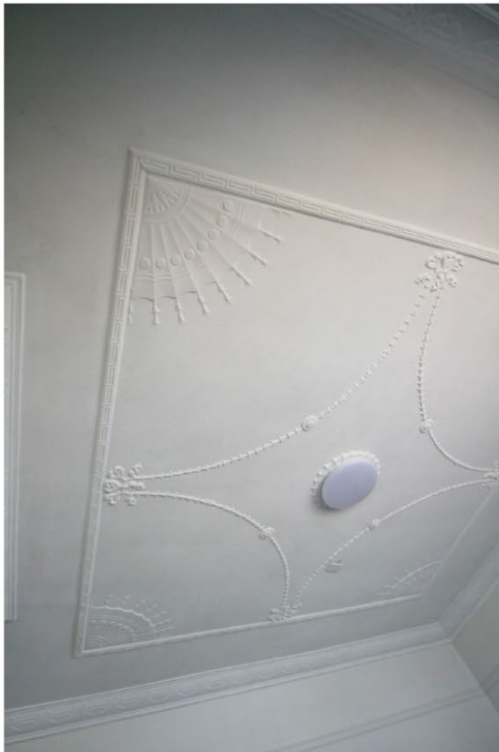
Figure 8. This photograph shows that Inter War decorative ceilings and cornices replaced the original Victorian ceilings and cornices.
