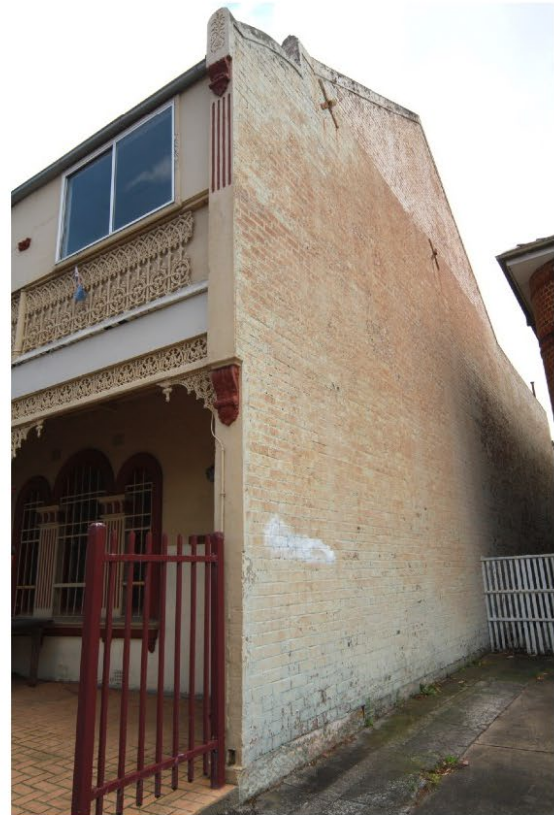
4.View of the eastern facade, showing the original wall of the principal building form and the rear wing.
