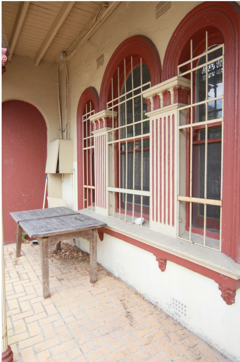
Figure 4. View of the front facade showing the recessed arch in the verandah end walls, the group of arched topped windows with Italianate moulded detail and cast iron wall vents in the upper section of the wall.
