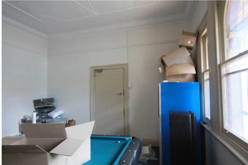
Figure 7. View of the ground floor front room, eastern wall. The interiors of the ground floor have been extensively altered and contain very little of the original building fabric. In this room the double hung window and architrave appears to be the only original building fabric.
