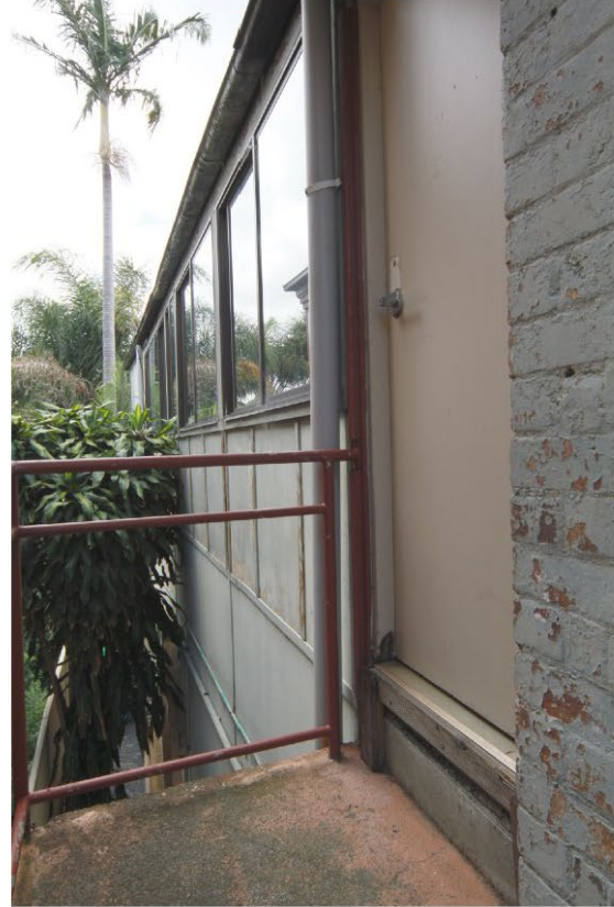
6. View of the first floor landing where the rear wing was extended in an addition to the property, which has light weight cladding and aluminium framed sliding windows.
