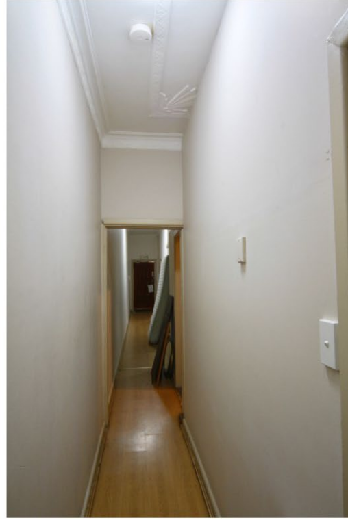
14. View from the ground floor corridor in the rear wing looking towards the front door:
