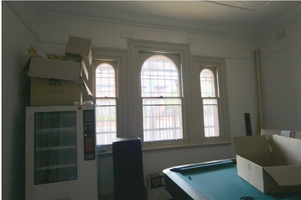
20. View of the front room on the ground floor noting the original ground floor windows.
