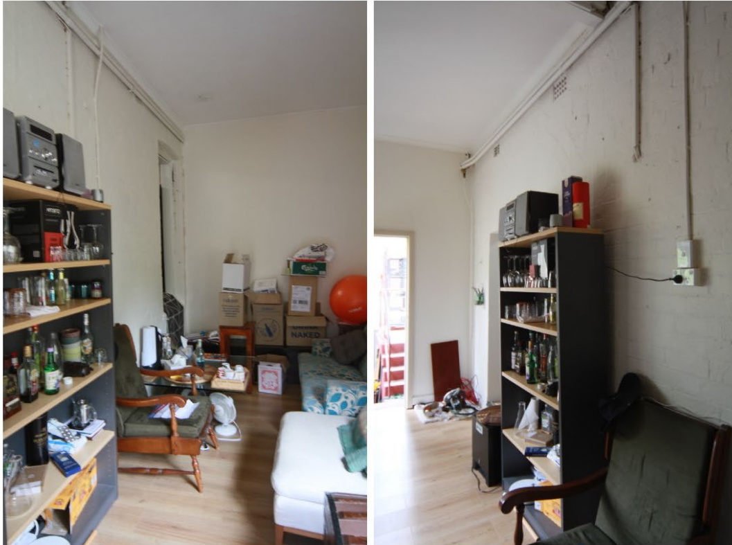
21 & 22. View of the ground floor rooms added to the western side of the original rear wing. The western wall of the rear wing and part of the joinery exists as shown in the first photo.
