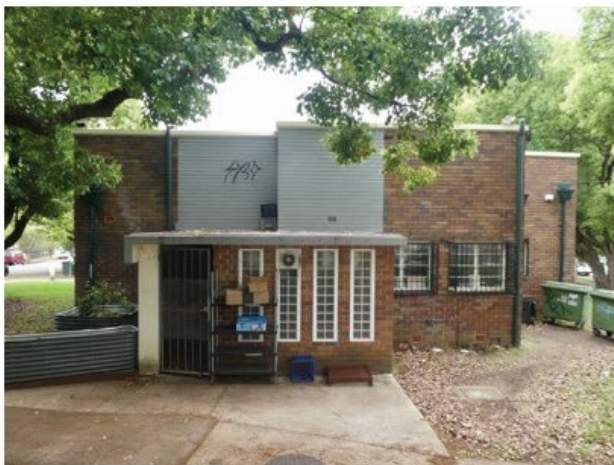
The building from the south. The walls above the rear service rooms have been painted since 2017, apparently by a Council contractor in an attempt to deal with damp issues.
