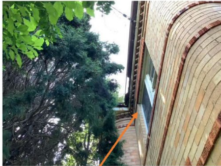
Damage to the roof and gutters.
