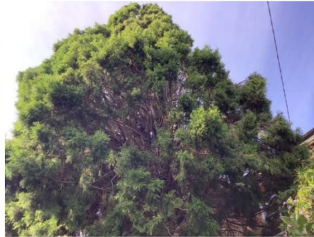
Canopy rubbing on the roof.
