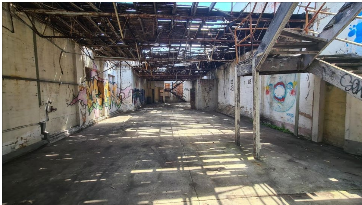
Figure 4: Internal ground floor view of subject site (No 33, Chalder Street) looking towards rear (Corona Projects 2021)
