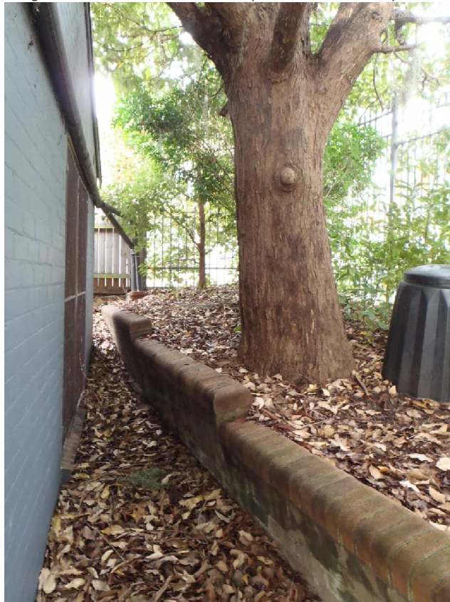
Figure 15. Photo T4. Brick wall displacement visible in photo.
