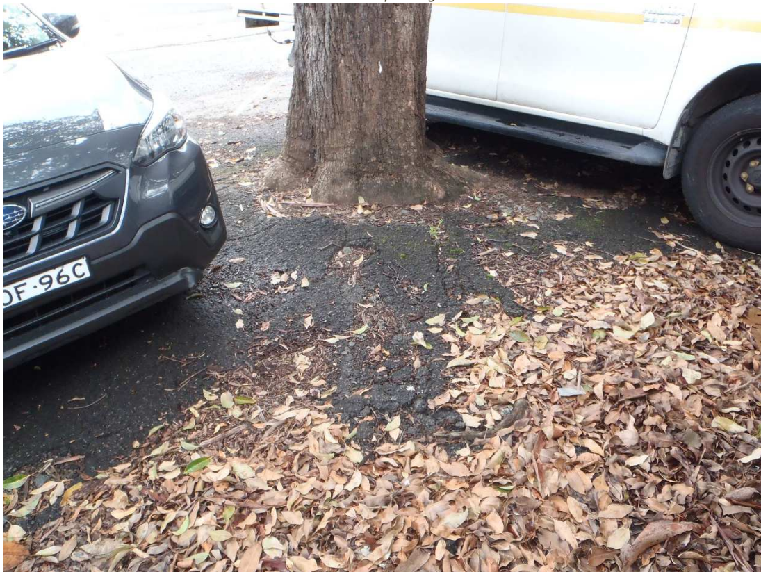
Figure 19. Trees 7-15 all within asphalt. Much displacement of the hard pave around the root crown base, rubbish dumped and cars parking.
