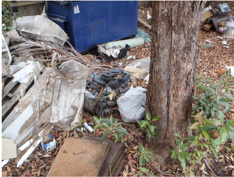
Figure 22. Tree T9. Slight stunting to tree. Rubbish dumped at base. Davies Lane in background. Tillandsia growing on limbs. Fungal mycelia present on trunk. Vertical split in trunk.
