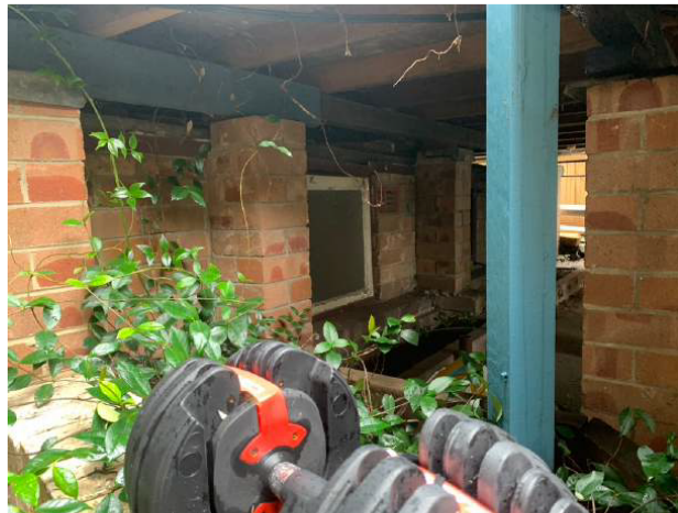
Figure 22: Looking under the deck towards the western wall of the basement. This is Post World War II brickwork.
