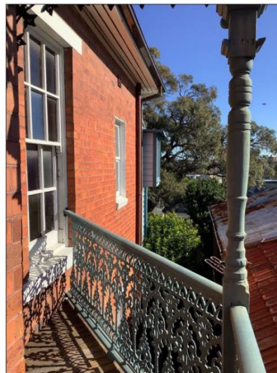
Figure 13: Detail of the balcony on the northern side at first floor level.
