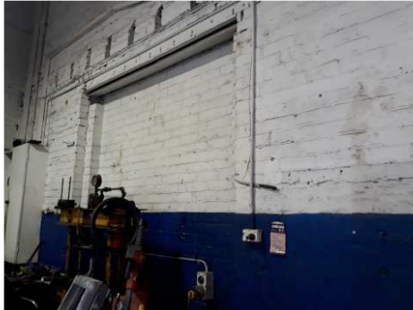
Figure 7.2 Infilled opening to the west side of the building to be reinstated
