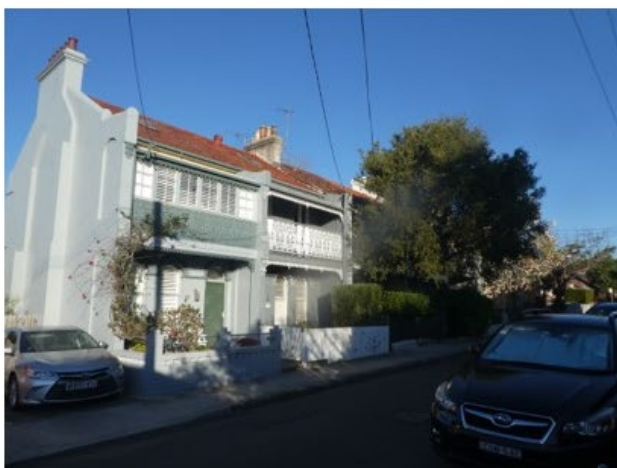
The terrace row from the north-west. No. 49 demolished, leaving No. 47 with end wall, chimneys and blocked fireplaces rendered and painted, and veranda enclosed.
