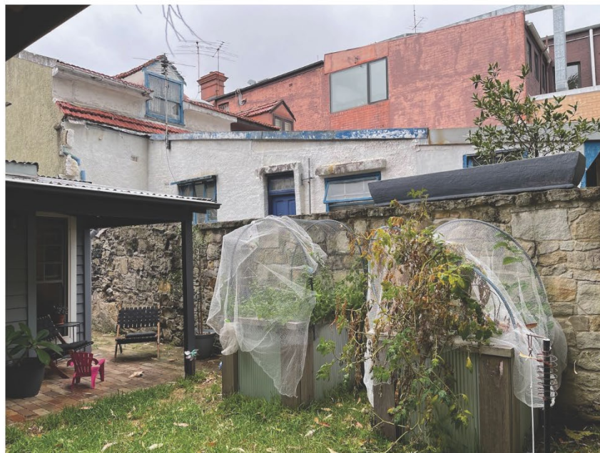
View to west side boundary wall with random rubble sandstone boundary wall.
