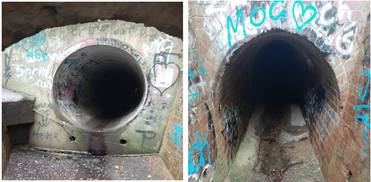
Figure 20: Reinforced concrete pipe culvert (top) and brick culvert (bottom) adjacent to Hercules Street containing potential microbat roosting habitat
