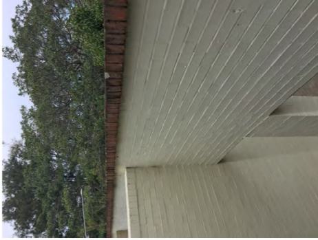
Existing painted brick and face brick capping to be retained on curved wall.
