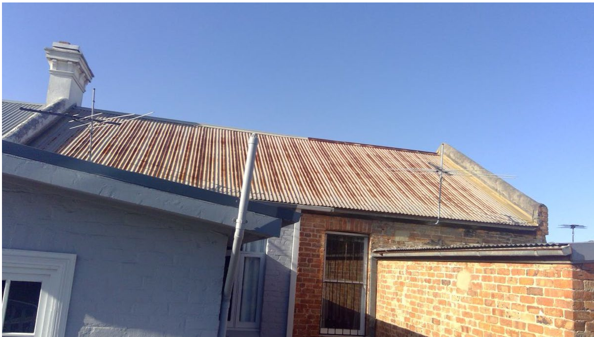
Photo 3: Photo of existing rear roof plan where rear skillion dormer to be located. Photo taken from rear first floor verandah looking south.
