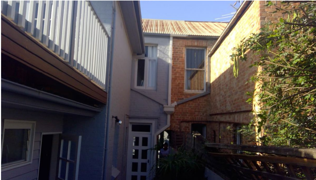
Photo 2: Photo taken from rear courtyard of site looking south, 86 Rowntree is the property on the left (light grey)
