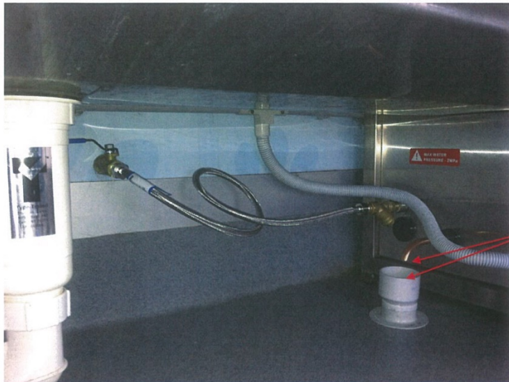
Tundish with air gap between the copper pipe and tundish highlighted. Only required for on board Storage Hot Water Unit
