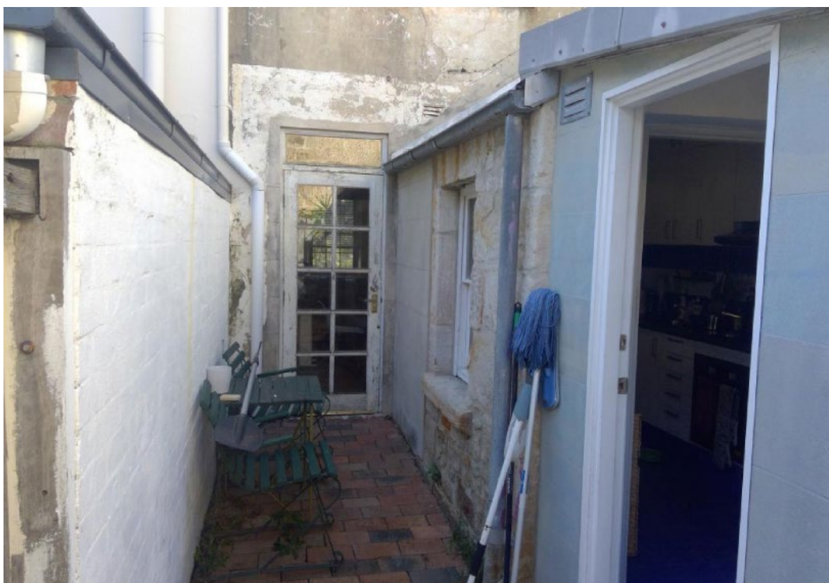
Figure 4: View of the property looking towards the eastern end from the rear yard.
