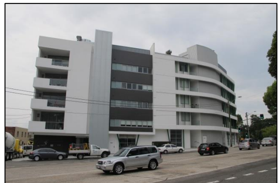
Photograph 8: 5 storey mixed-use development under construction at No. 118 Old Canterbury Road with an FSR of 2.67:1, as viewed from Old Canterbury Road.
