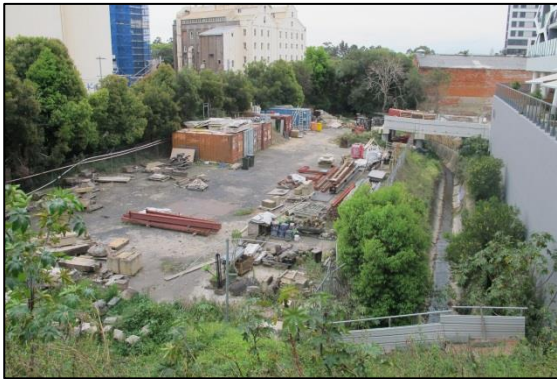
Photograph 3: The subject site as viewed from Old Canterbury Road, with the storm water channel to the east
