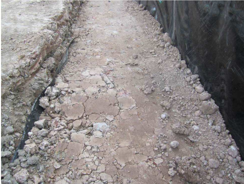
Figure 30 Compacted clay liner – note 1m depth of clay liner on trench face on left hand side of photo
