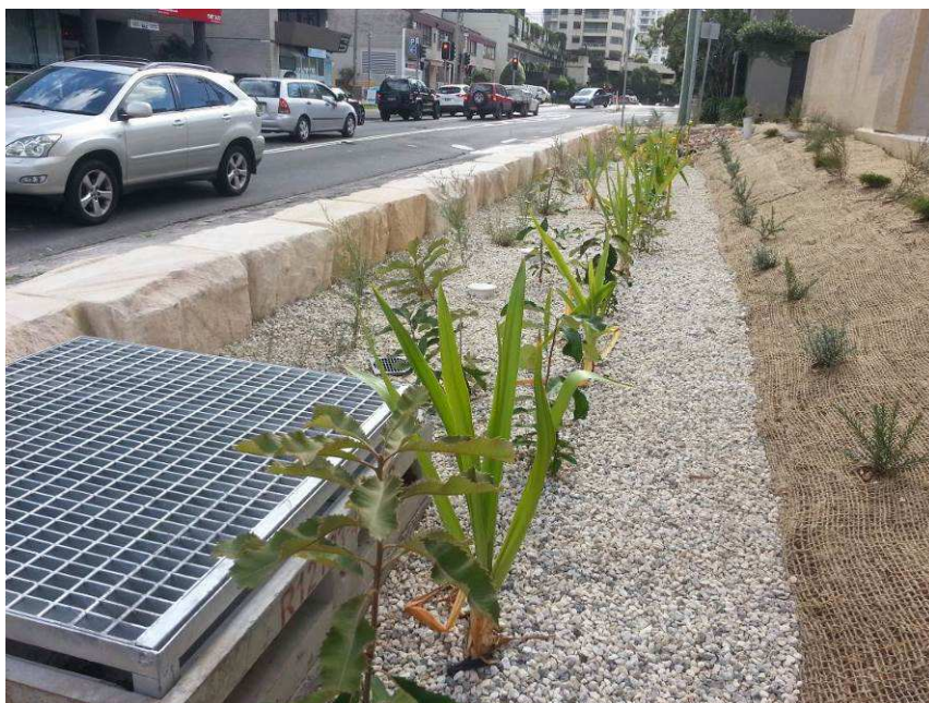
Figure 15 Clean no fines rock mulch to base of rain garden and jute mesh to batter slopes
