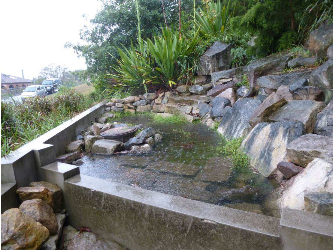
Figure 13 Coarse sediment forebay
