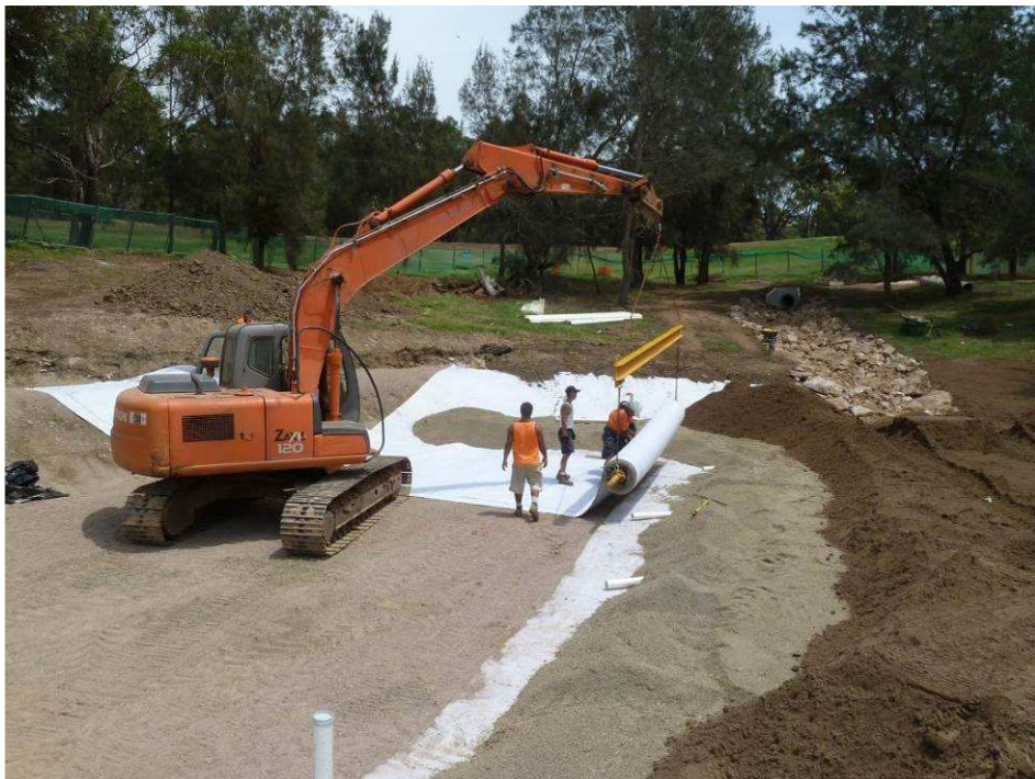
Figure 29 Geosynthetic clay liner being installed (note preparation of subgrade below liner which is free of any irregular rocks or sharp material)
