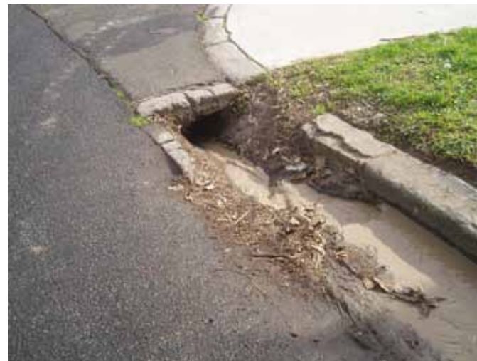
Sediment escaping from building sites enters into the stormwater system that discharges to the Cooks River.
