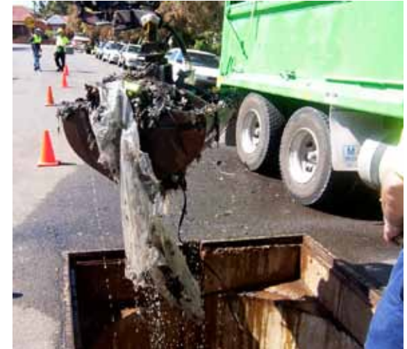
Cleaning out the CDS unit in Balfour Street that traps some gross pollutants heading for the Cooks River.
